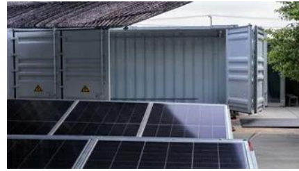
Advantages and disadvantages 50kW photovoltaic container
