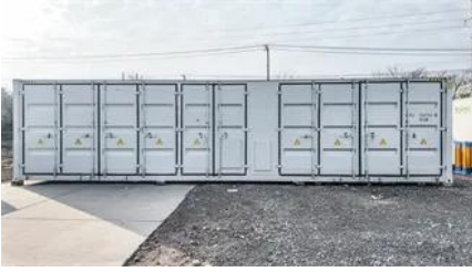
Cameroon information engineering new energy storage project
