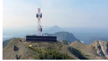
Hybrid energy isolation lightning protection system for solar container
