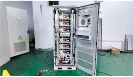
Battery Storage As A Service Iceland , ESAFETY SOLAR CONTAINER
