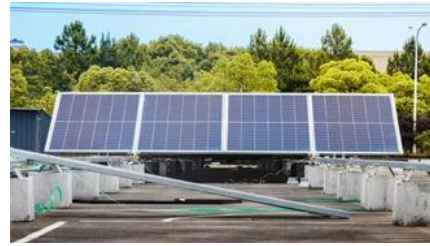
Honiara solar container communication station inverter grid
