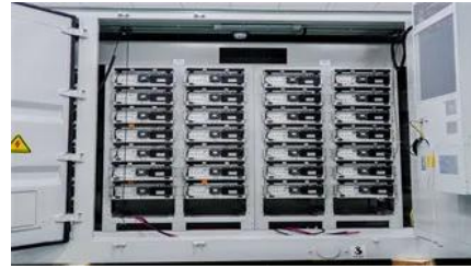
Kigali solar Energy Storage Inverter
