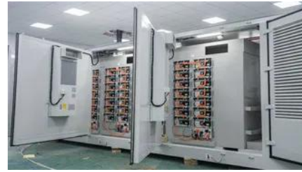
Earthquake Monitoring Photovoltaic Energy Storage Station
