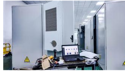
Namibia's Battery Energy Storage System Production: Powering a
