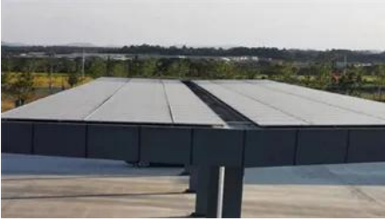
Outdoor Communication Base Site R01 - Modular Power Station for
