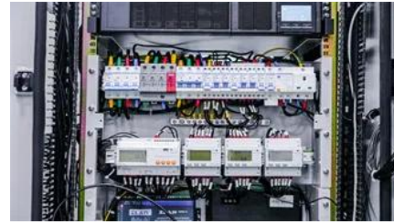
150-foot photovoltaic energy storage container for subway stations
