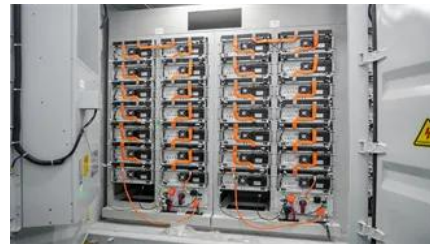
UPS Power Supply , 4 set 150kWh Solar Systems in the Philippines
