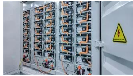
Bess Solar Battery Energy Storage System 5mwh
