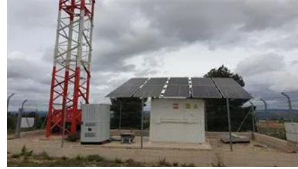
Solar-Powered Container House: Complete Off-Grid Energy Setup
