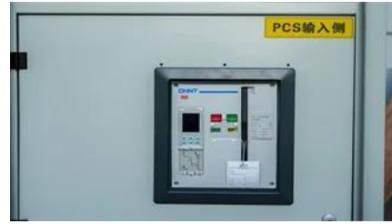
Energy Storage Cabinet, energy storage system, New Energy
