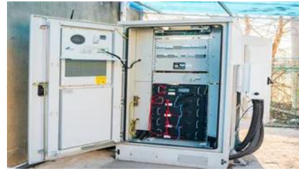
Vanuatu Solar Power Generation and Storage System Home
