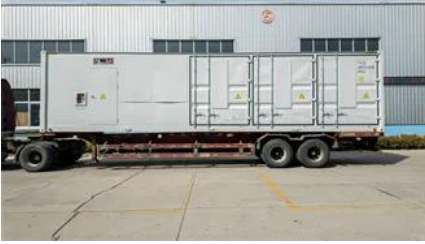
Port Louis solar energy storage cabinet solar container lithium battery
